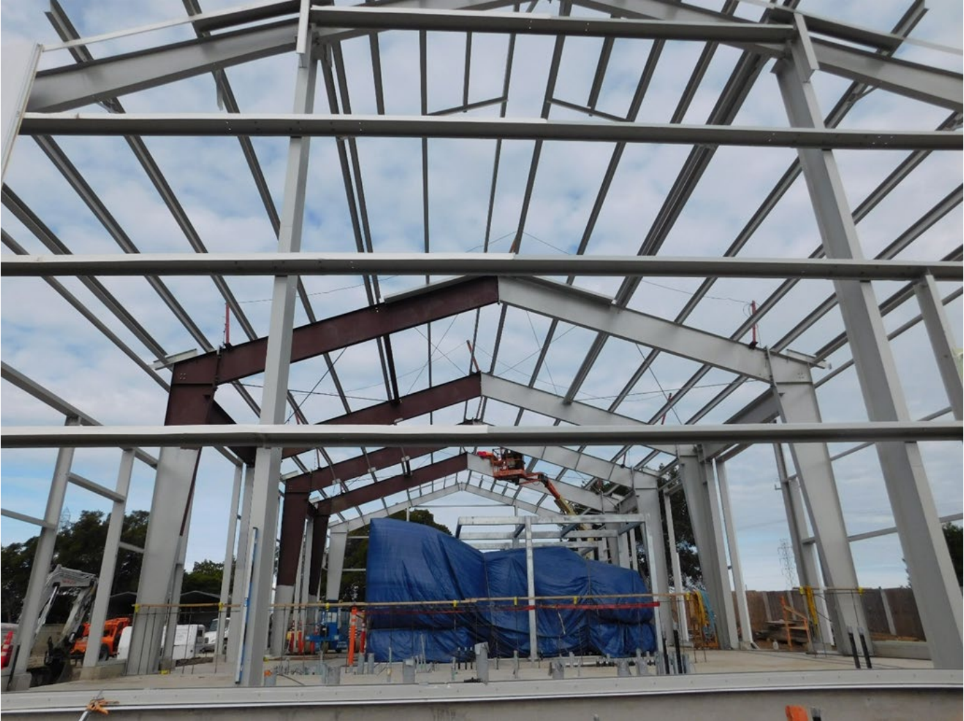
New Standby Power Building
