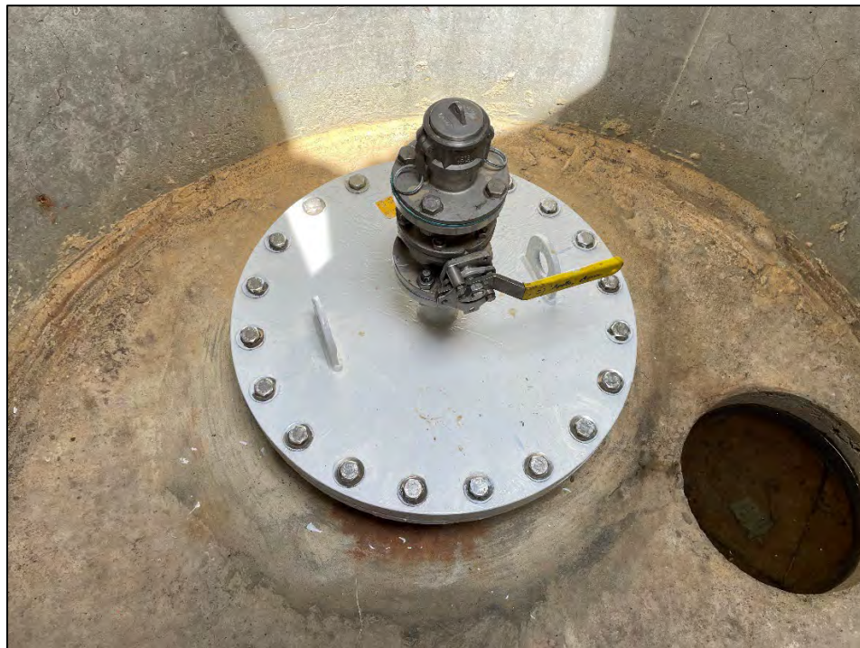
Figure 3 – Before and after photos of the new valve and pipe flange cover at the Boyce Road Access Manhole
