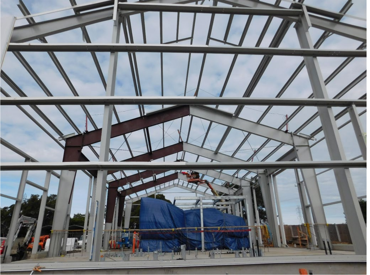
New Standby Power Building
