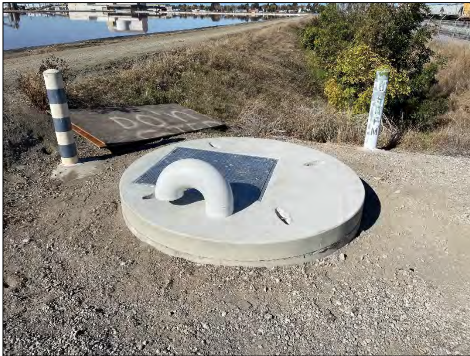
Figure 6 – Before and after photos of the new access cover and hatch at the Cargill Salt Fields North Access Manhole
