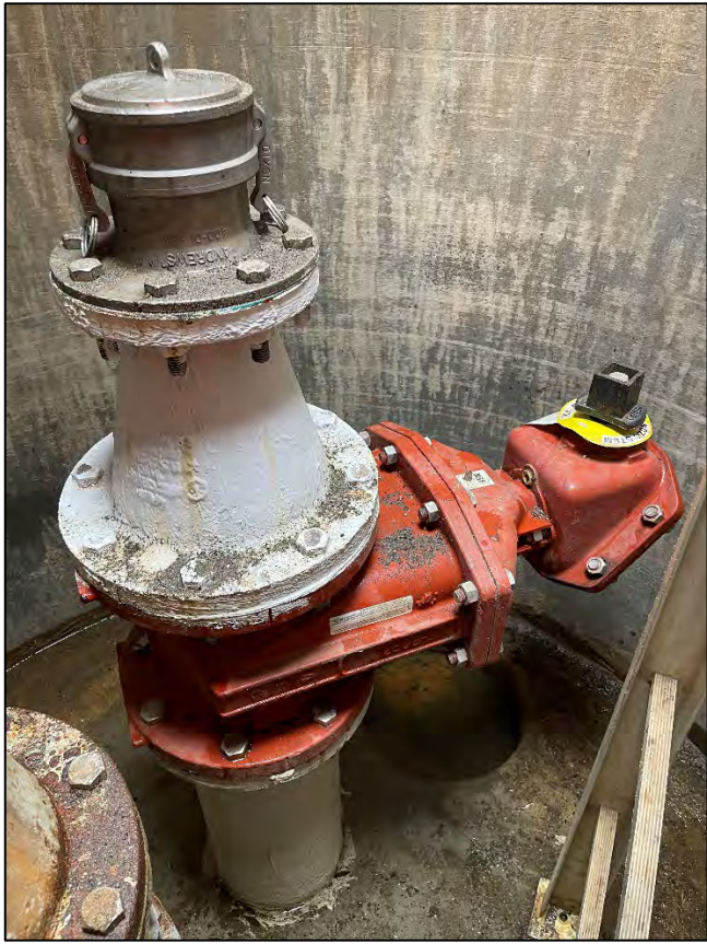
Figure 4 – Before and after photos of the new pipe connection and valve at the Cherry Street Blow Off Manhole
