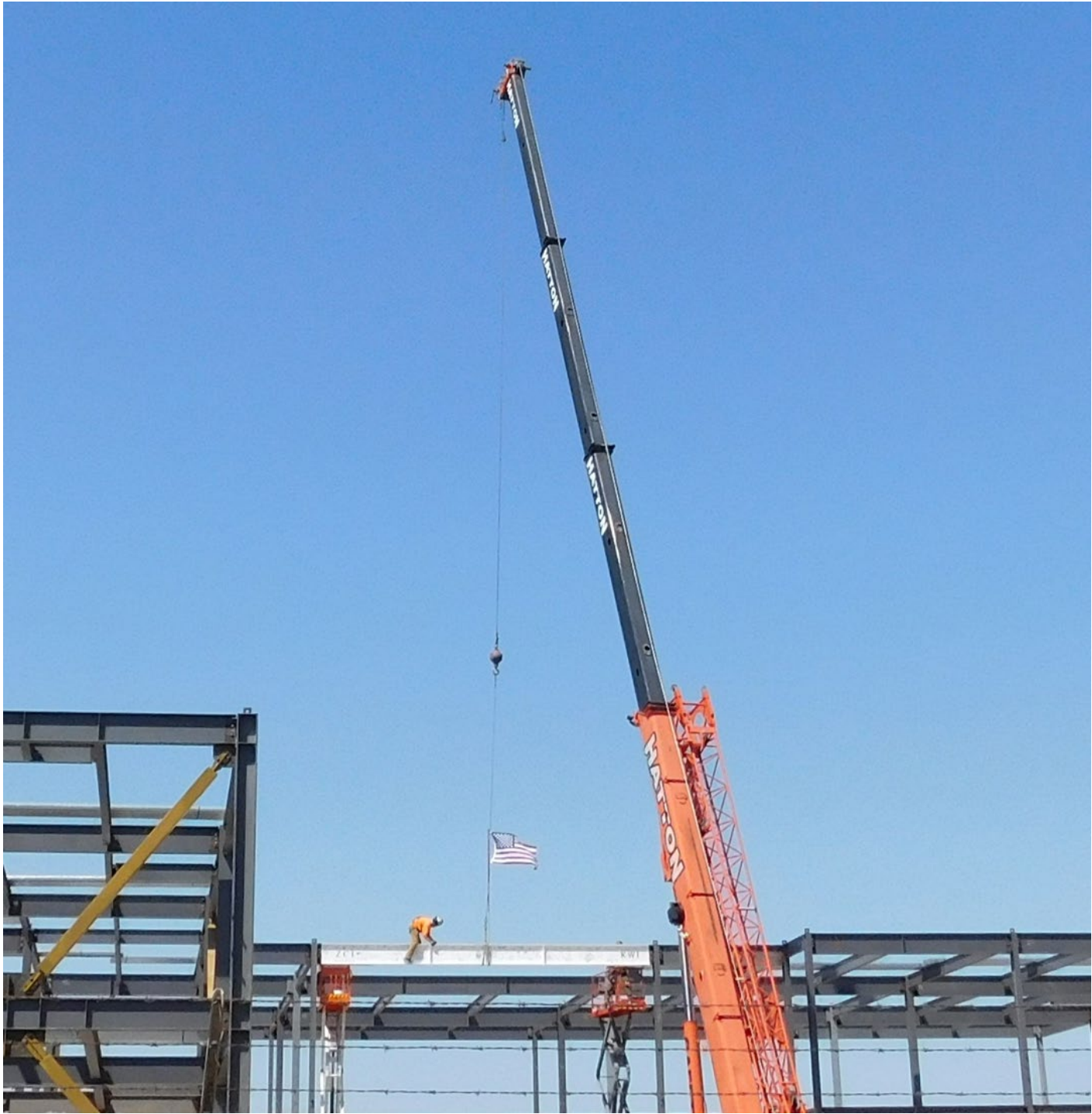
Placement of the Topping Beam on the New Campus Building Cover Picture: ETSU Aeration Basin Construction
