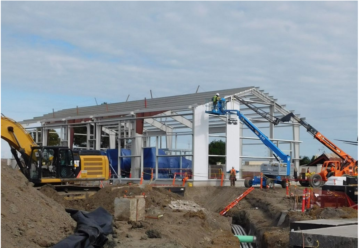
New Standby Power Building
