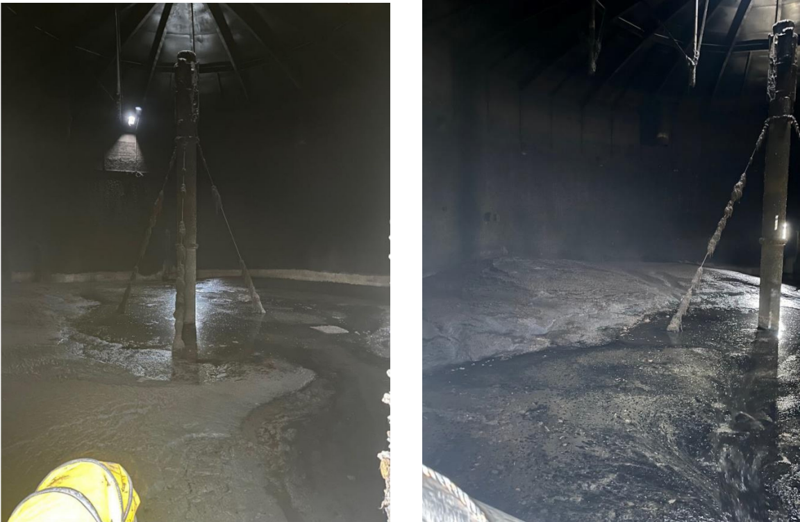
Figure 1 –Interior Pictures and Dimensions of Primary Digester No. 6
