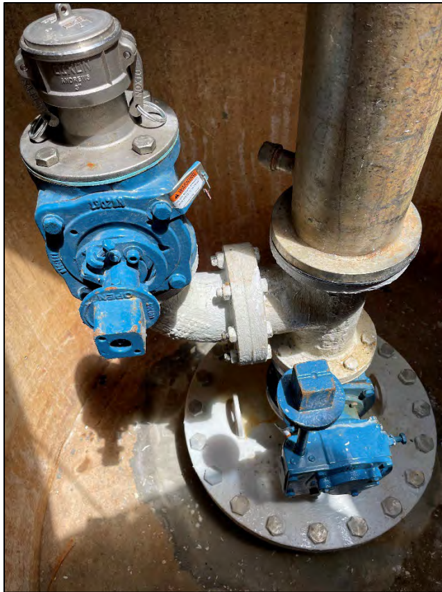
Figure 5 – Before and after photos of the new valves and pipe flange cover at the Auto Mall ARV Manhole
