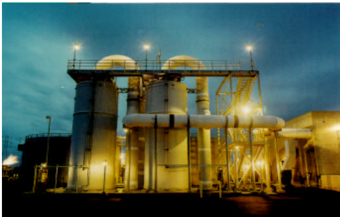
Union Sanitary District's "Odor Scrubber," which reduces smells.
