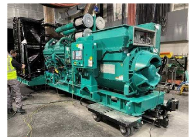
Standby Power Generator
