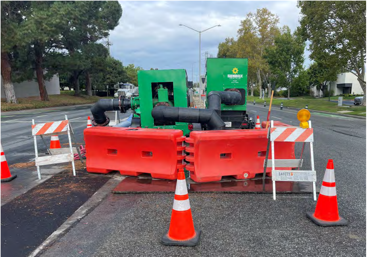
Figure 2 – Temporary Bypass Pumping System
