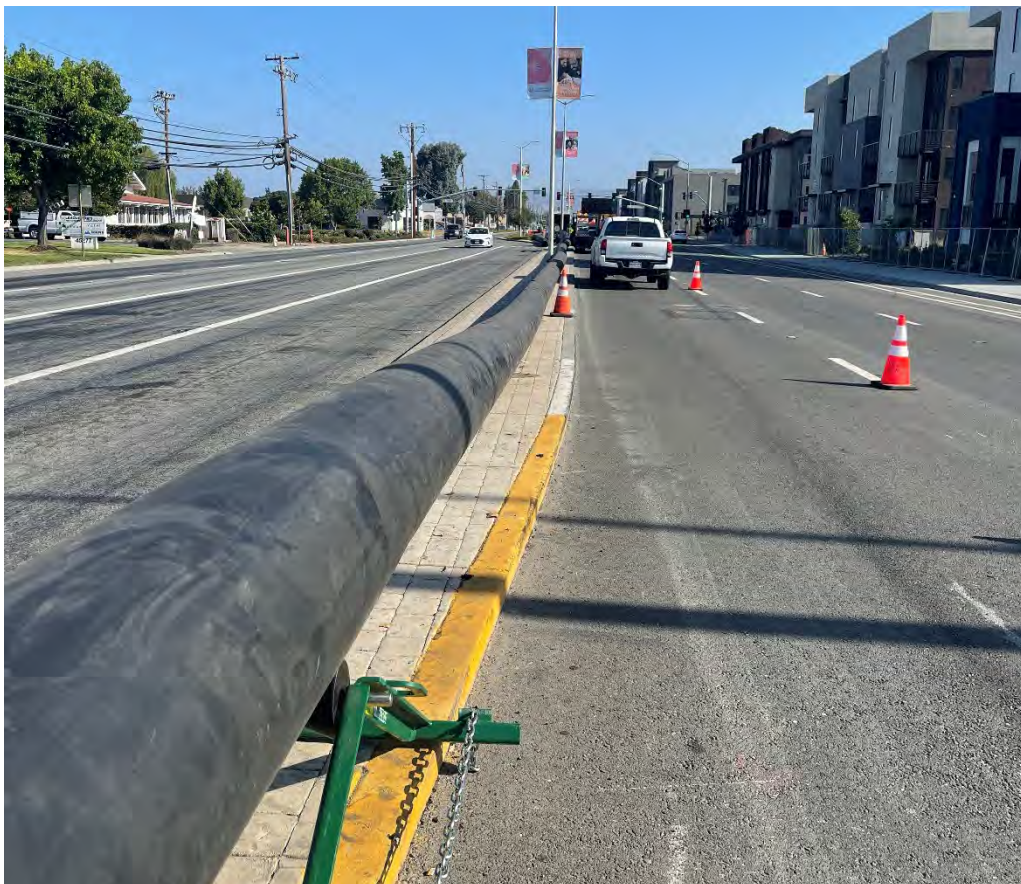
Figure 5 – Bypass Piping Routed on Center Median
